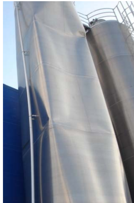
Figure 1. Postbuckling shape of silo with internal underpressure (photo: anonymus)
